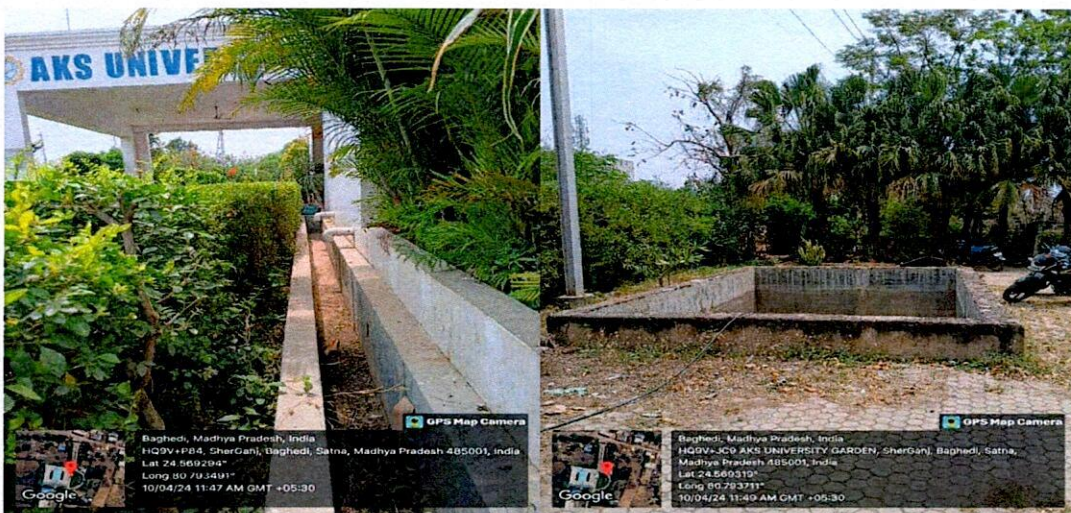
Figure 2: Rain water storage tank (A Block)
