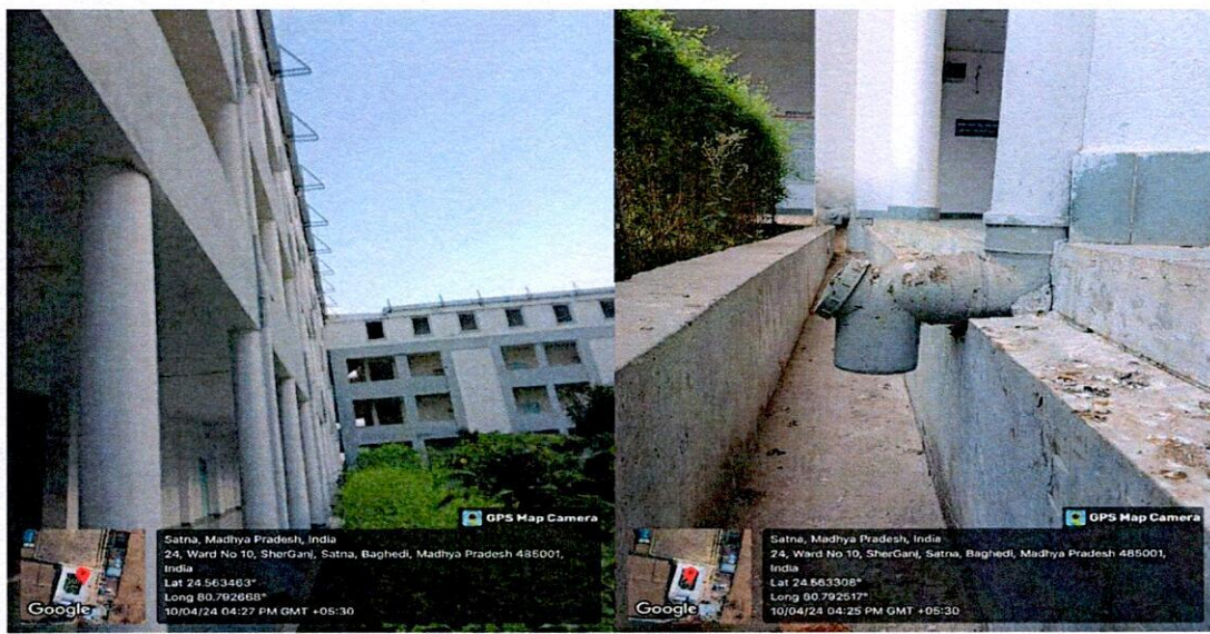
Figure 5: Rain water harvesting (C & D Block)
