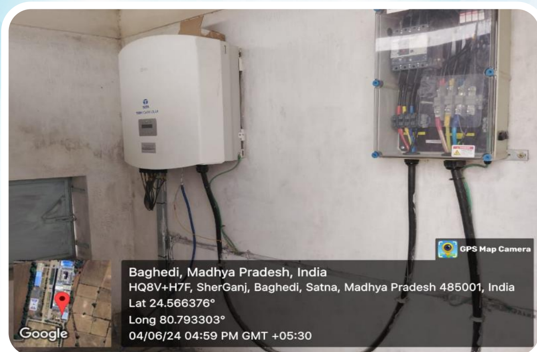
Photo 3: Photo- Inverter D -Block
