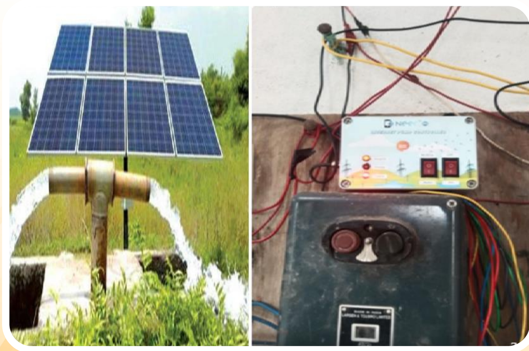
Photo 7- Sensors based motor switch for Solar Submersible pump
