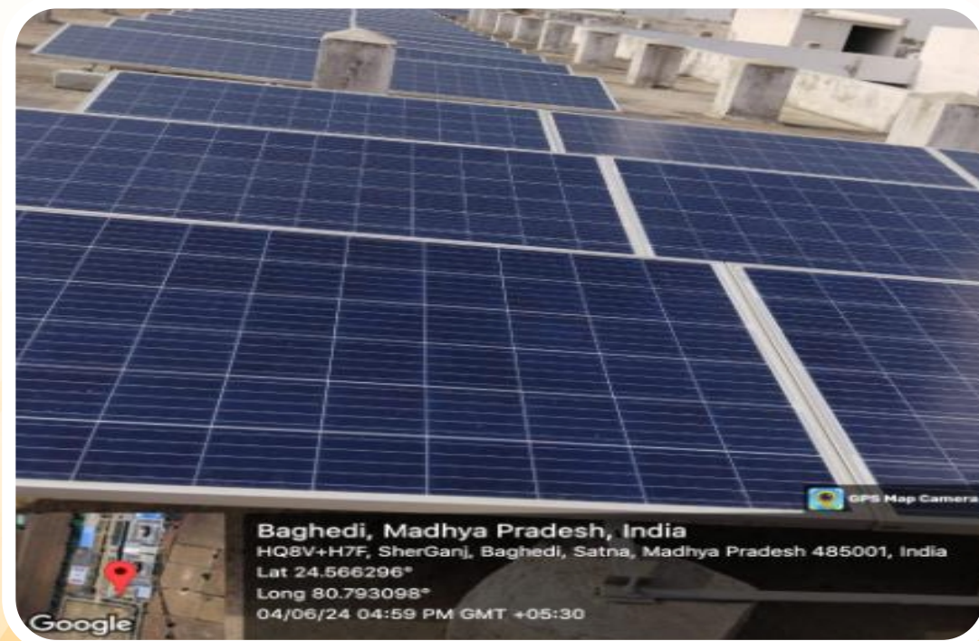
Photo 4: Photo-Solar Pannel D block
