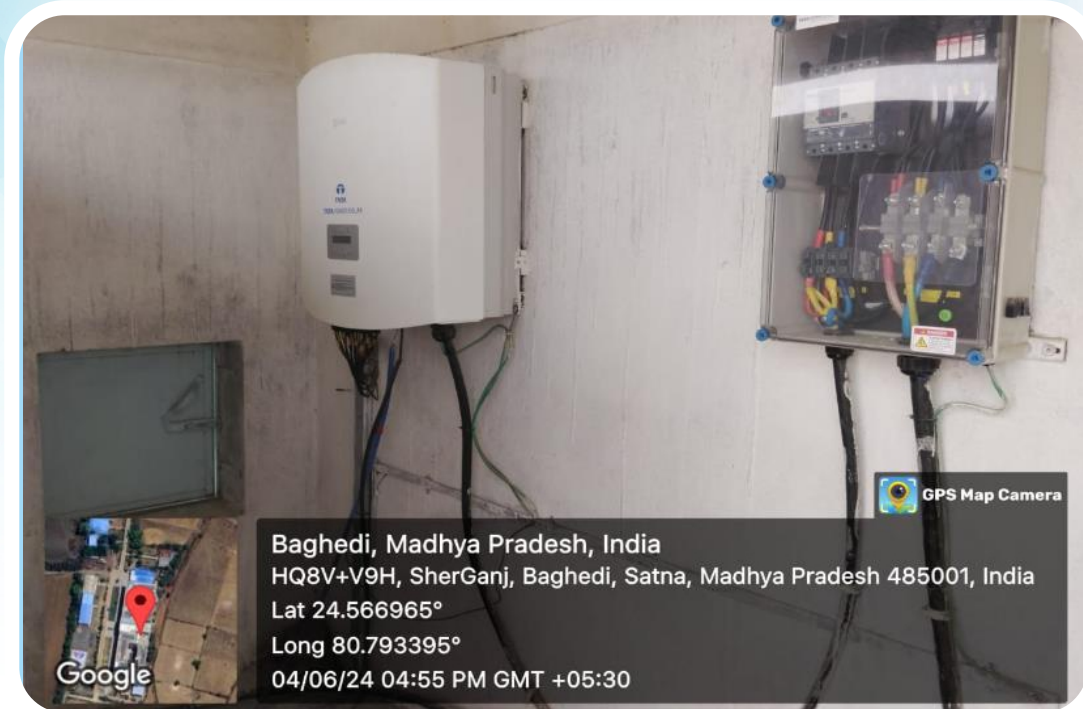
Photo 1: Picture-C block Inverter
