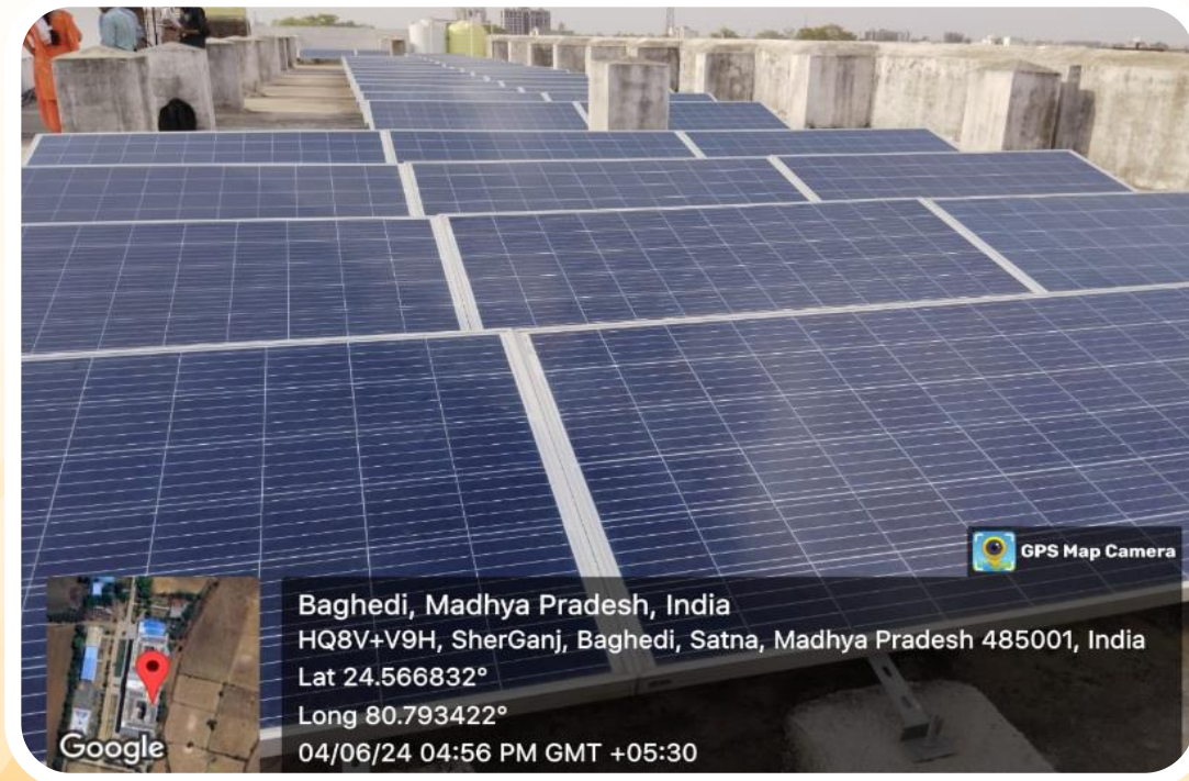
Photo 2: C Block Solar Panel section
