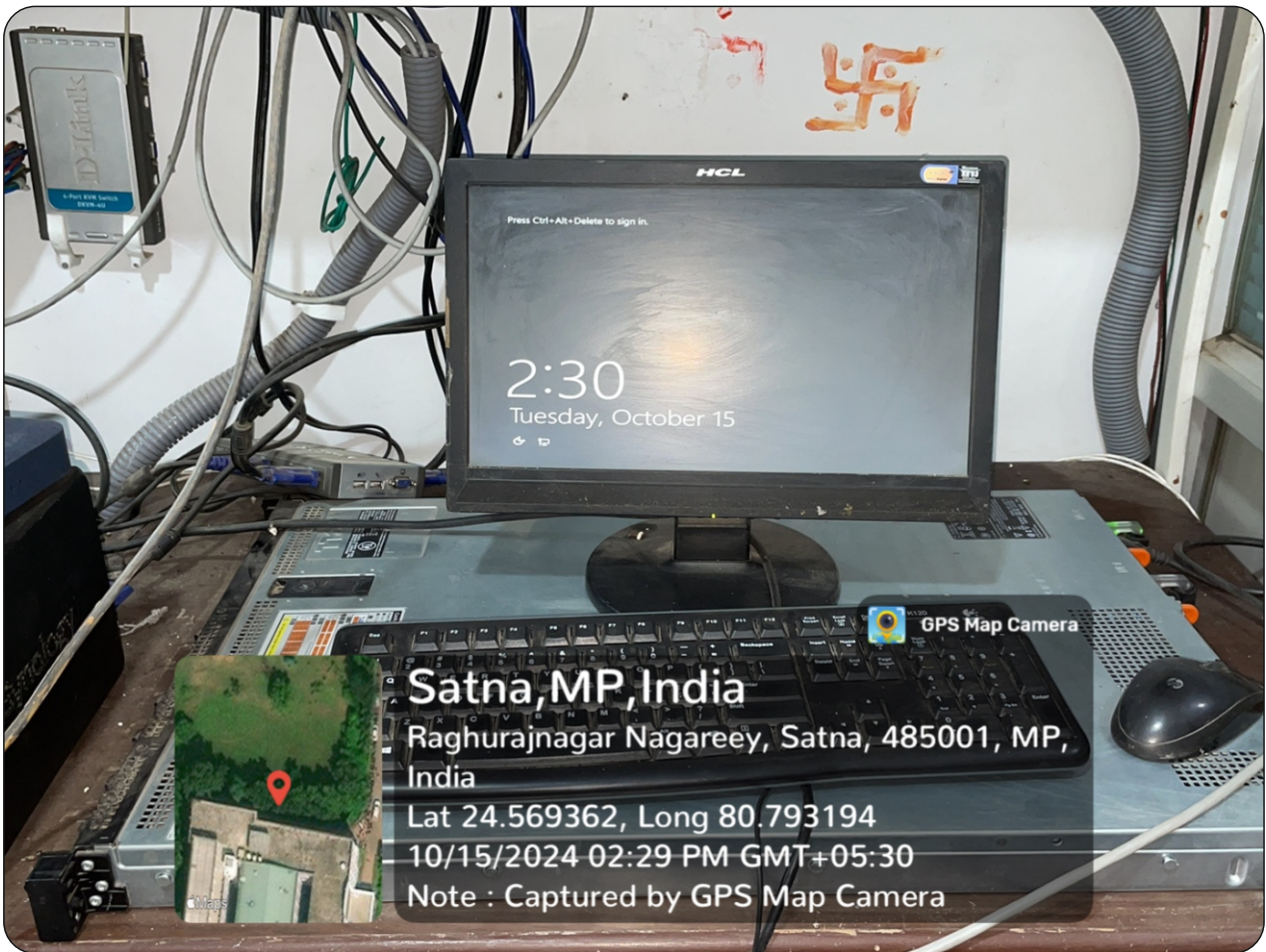
DELL RACK SERVER
