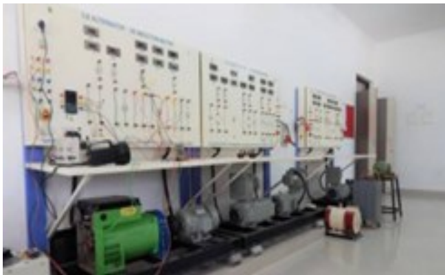
Electrical Instrumentation Lab
